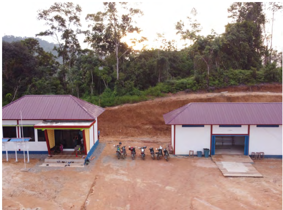
Construction of AMB infrastructure has started in early July 2023, the construction was completed in December 2023 © WWF Indonesia
